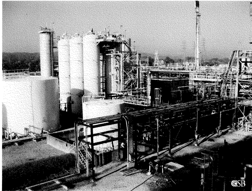
Figure 6: View of the MIC storage tank in the Methomyl/Larvin unit showing the blast blanket first installed in 1982 and then extended upward in 1994.
