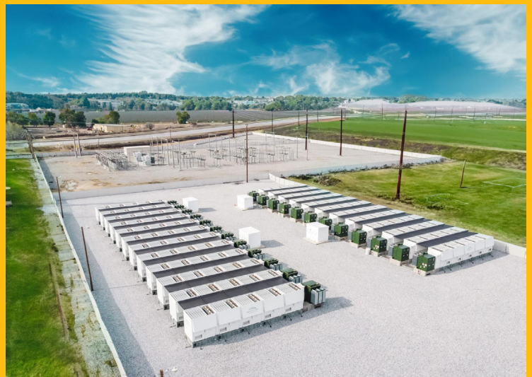
MICROGRIDS FOR RELIABLE BACK-UP POWER IN TEXAS. SOURCE: ENCHANTED ROCK
