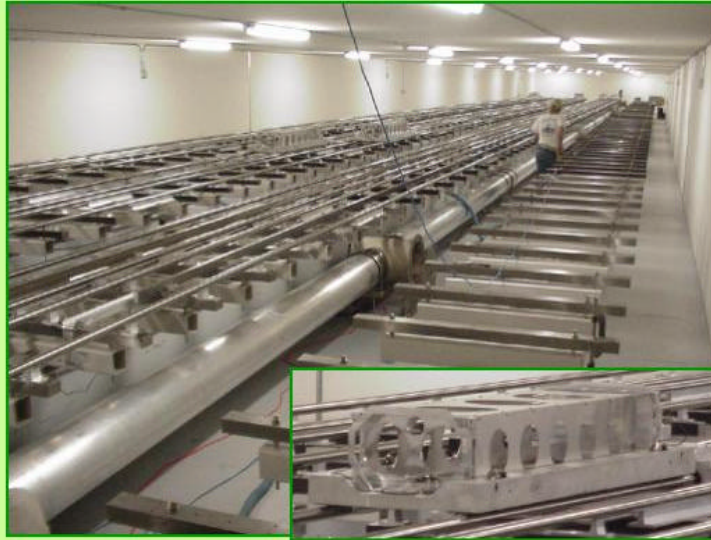
Figure 1 11 The inside of the OPLE building of the CHARA Array. On the left are six sets of optical delay lines. The inset shows one of the delay line carts. The right most pier has been left empty, until additional telescopes are built.
