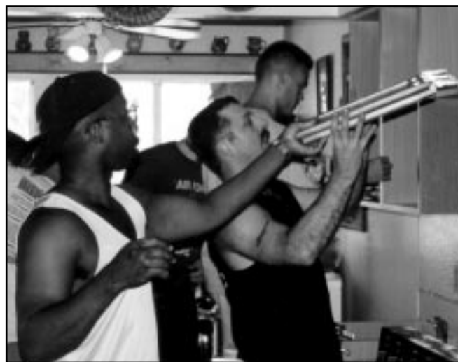
Front, Tech. Sgt. J.T. Williams and Master Sgt. Jim Welker, 692nd ISS, work hand-in-hand installing new kitchen cabinets and doors.
